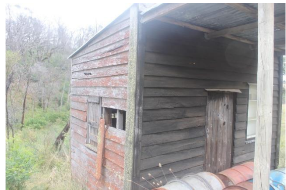
Sawmill outbuilding that survived the 2019 fire at Nerriga in NSW, Australia, showing the soot deposition on the side that faced the firestorm. Image: Alison Wain, 2019
