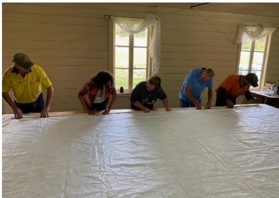
Peter van Diesen, Sabine Cotte, Nadine Fleischer, Phil Large and Kevin Fleischer installing the new hanging system on the treated Bullumwaal Hall stage curtain.
