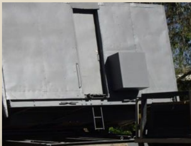
Figure 4 | RTA equipment housing before and after treatment.
