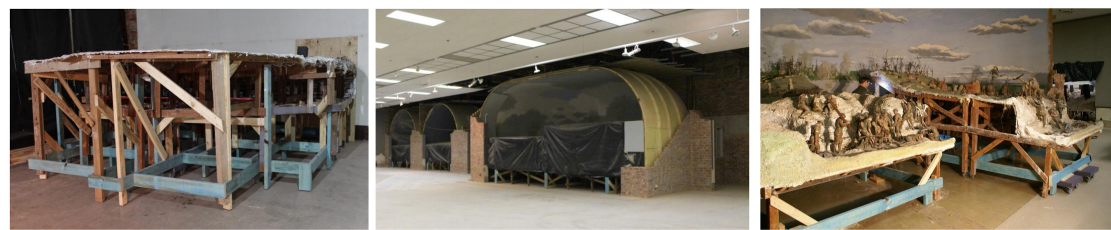
Additional reinforcement to base of dioramas; during demolition of non-structural 1970s walls; sectioning of Mont St Quentin to fit through doorway
