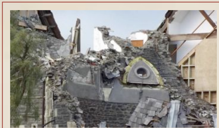
Figure 1 | Aftermath of the earthquake.
