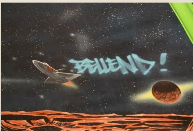
Figure 5 | Graffiti damage to the interior space-themed mural.
