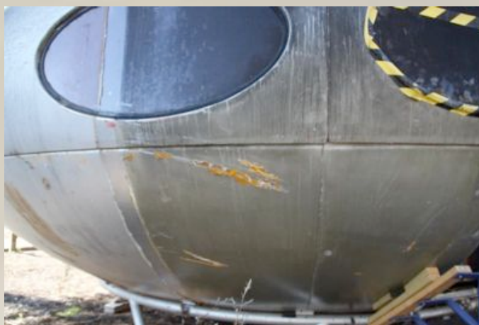
Figure 4 | Surface abrasions and damage to the GRP caused during transit. Soot staining from the fire.
