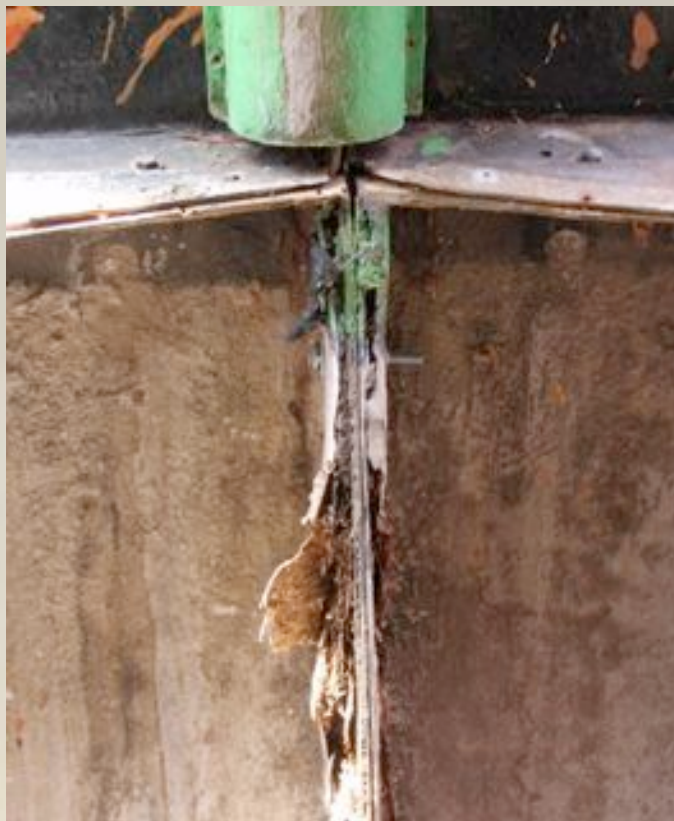
Figure 6 | Water damage resulting in swelling and breakdown of composite board on flanges.
